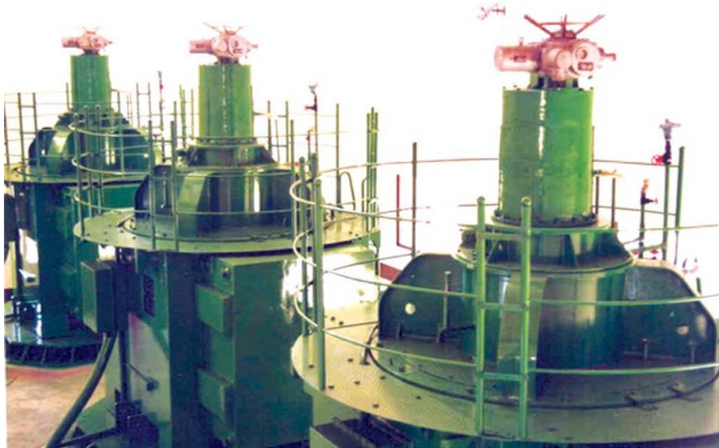
Plant and equipment of pump station
